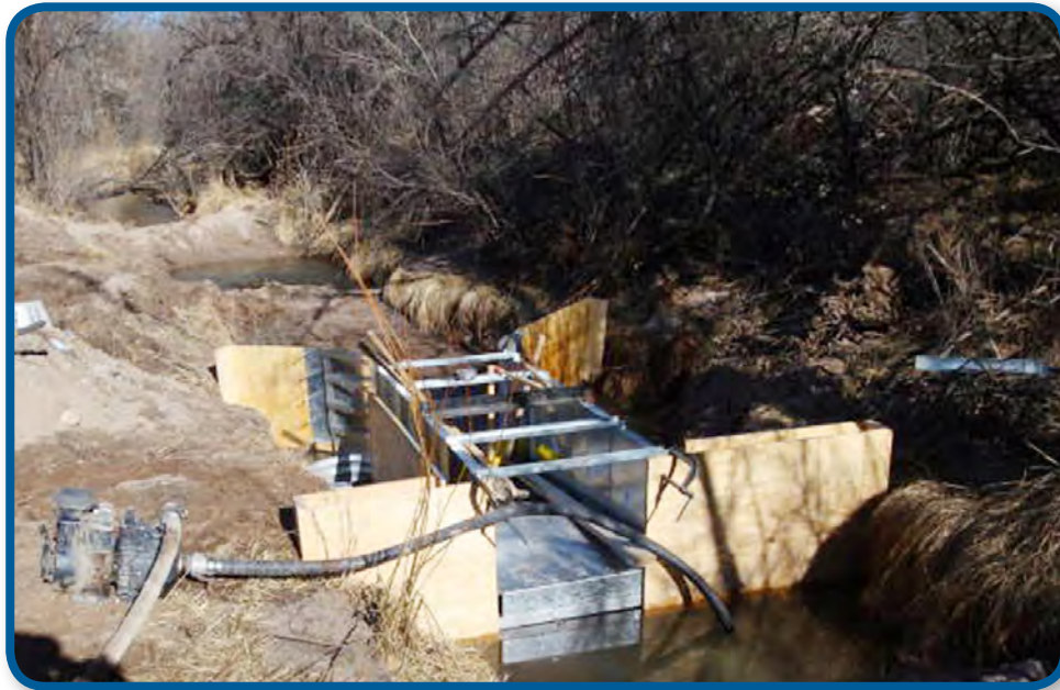
Framed Flume Pumping Bypass
