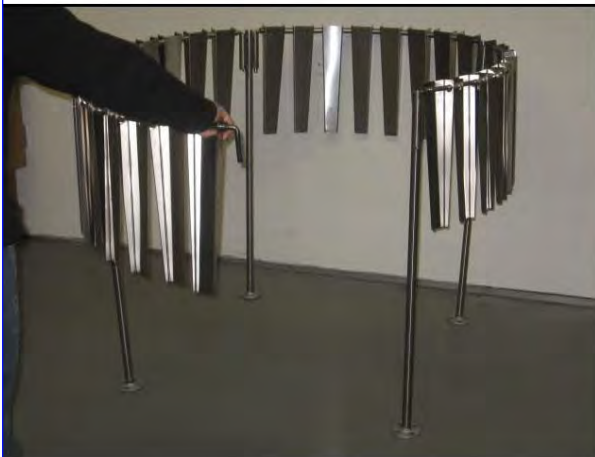
Photo 7 Windscreen gate quadrant swings open to allow access to rain gauge
