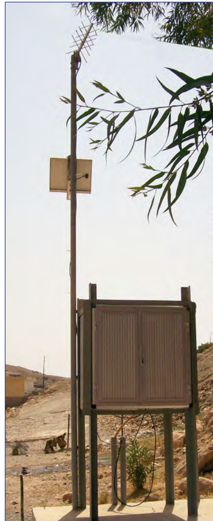
Sutron's Bubbler Station at Darbandikhan Dam, Iraq
