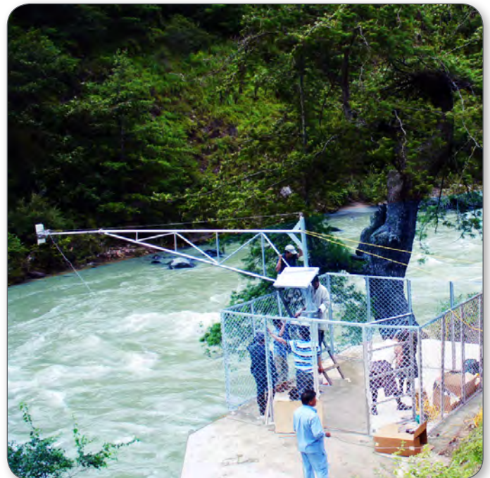
Tamchu Automatic Water Level Station (AWLS)
