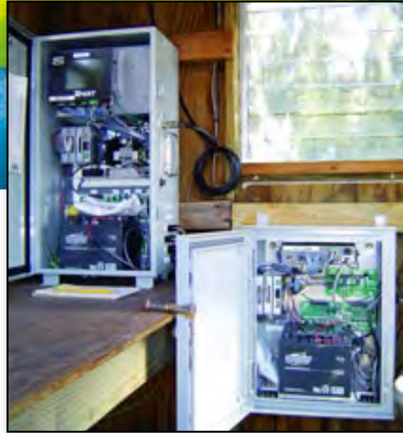
Sutron's NOS-Approved Main Station & Redundant Station Configuration, Pacific Warning Center, Hawaii
