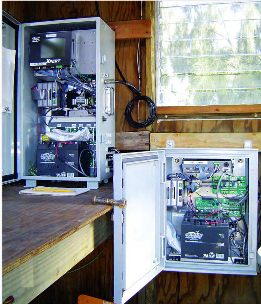
Sutron's NOS-Approved Main Station & Redundant Station Configuration Pacific Warning Center, Hawaii
