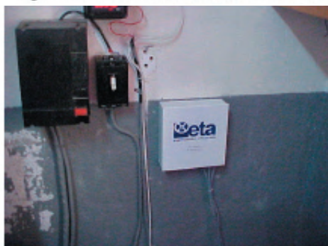
FIG. 5 SUPPLY AND BATTERY BOX
