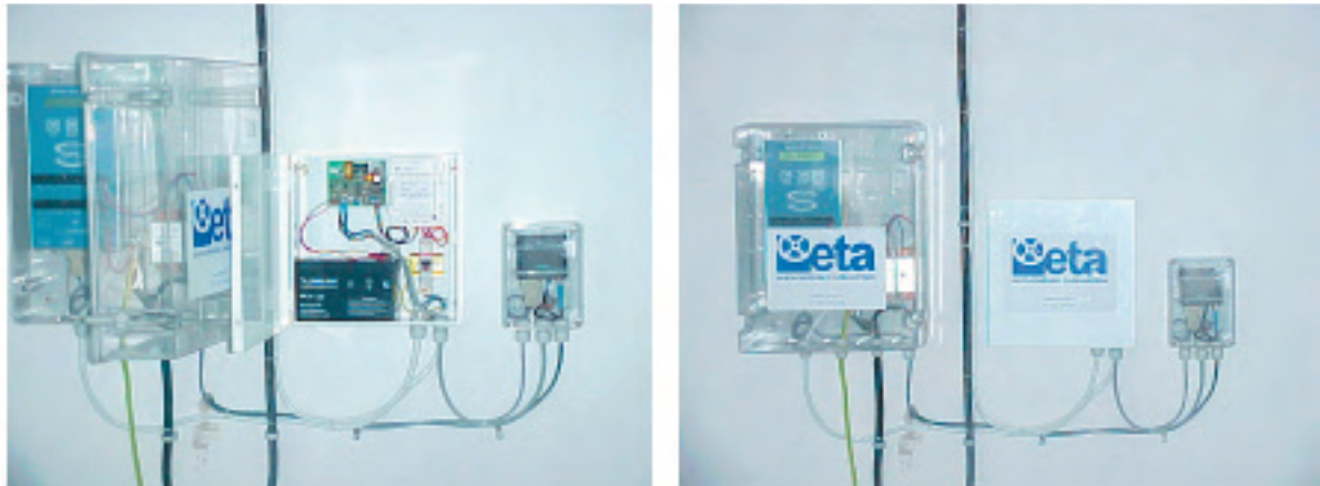
FIG. 4 - DATALOGGER 9210 XLITE, SUPPLY AND BATTERY BOX, MODEM SIEMENS MC35T. (HERCULANE DAM)
