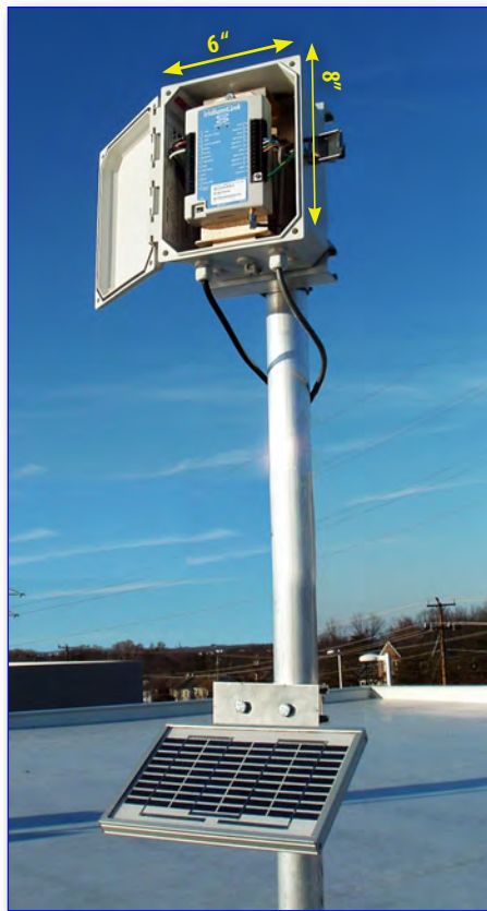
Iridium Station, Rooftop Sutron Headquarters
