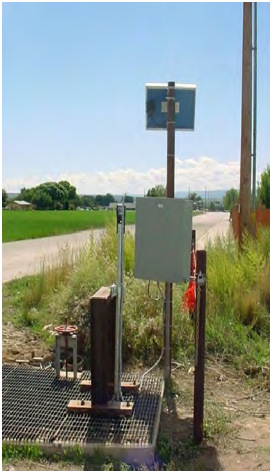
Typical DitchMaster® Station
