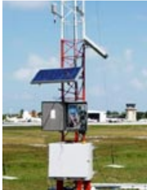
Sutron Airport Weather System Cayman Islands International Airport
